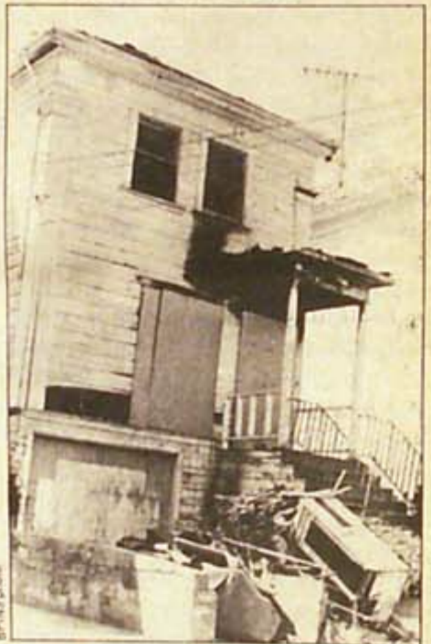
West Oakland residents are angry over illegally dumped garbage and fire trap abandoned housing.
